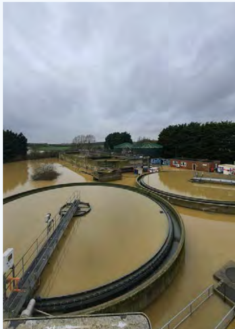
Anwick Water Recycling Centre under water, the source of one of our Category 2 pollutions.
