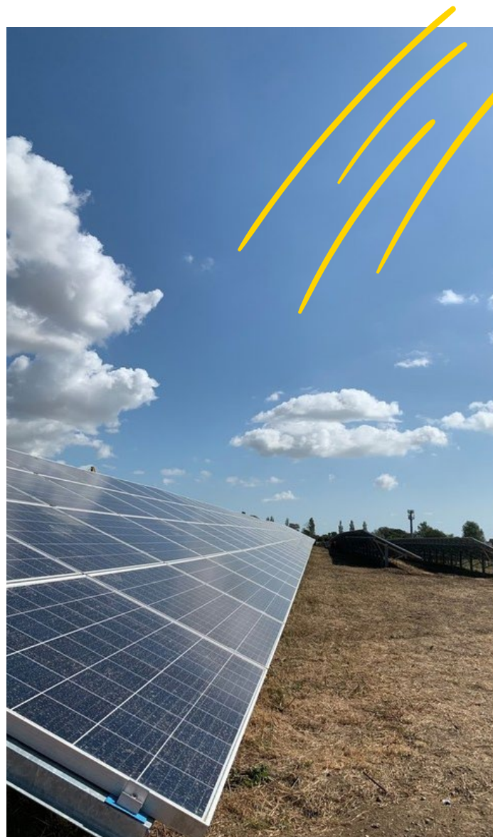
Anglian Water's 894KWp solar installation at Jaywick Water Recycling Centre meets up to 36 per cent of the site's energy requirement
